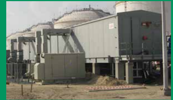
Stationary pre-fabricated electrical enclosure
